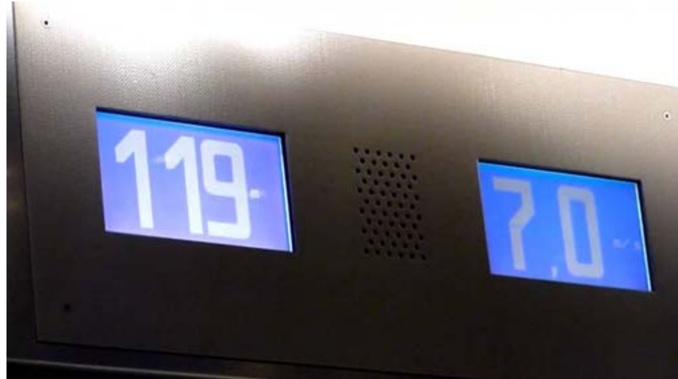
Fig. 3: Display of the lift cabin's actual height and speed in the Olympia tower in Munich. Source: https://youtu.be/0V6bJ0TUI
